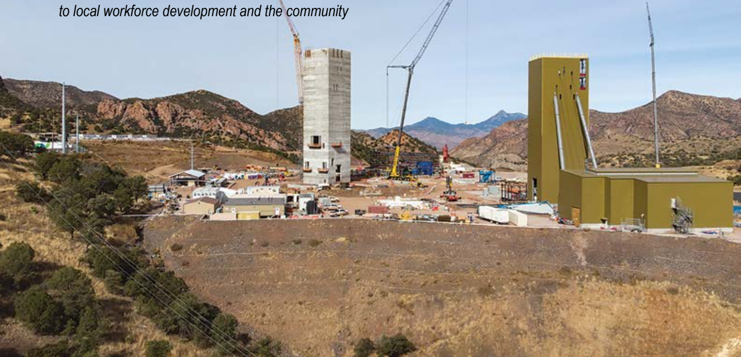
The headframe for the main shaft at the Taylor deposit was recently completed. (Photo: South32)
