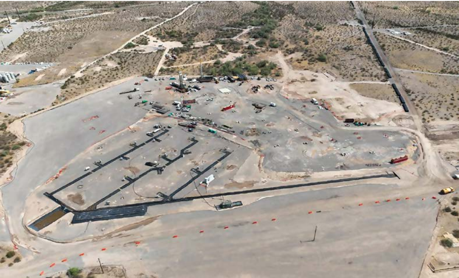
Two drill rigs and a development rig work on production wells. At the end of 2024, 51 production wells had been completed and a third drill rig is now operating at site. (Photo: Taseko Mines)
