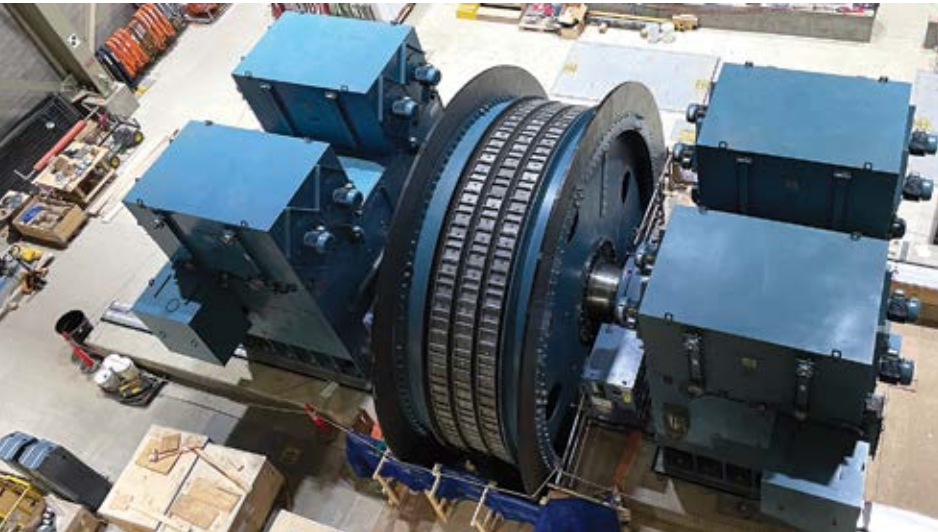
One of the friction hoists being installed at the Jansen potash project in Canada. (Photo: BHP Jansen)
