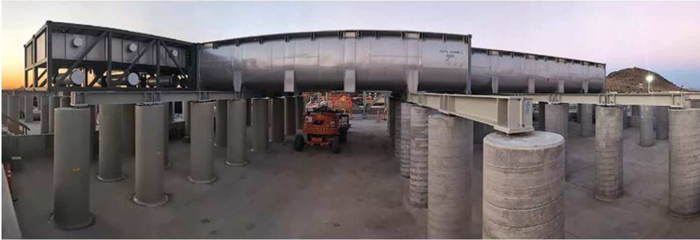
First solvent extraction settler and launder modules were placed in September 2024. (Photo: Taseko Mines)
