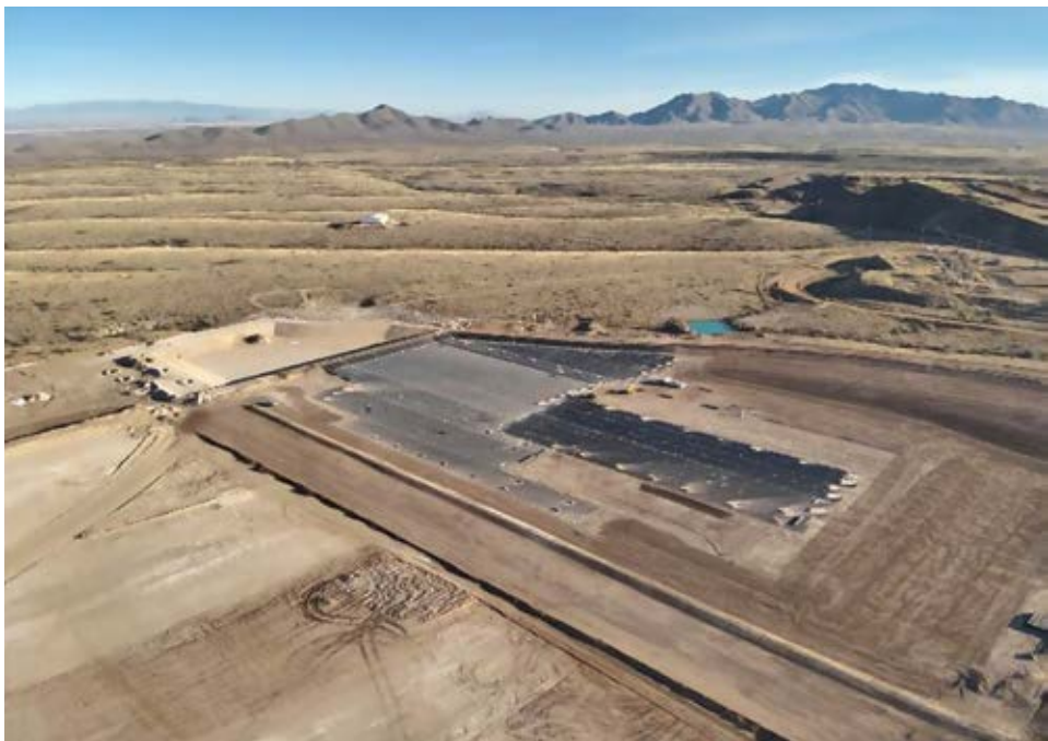
Gunnison started construction on a new leach pad for the Johnson Camp mine in August. (Photo: Gunnison)
