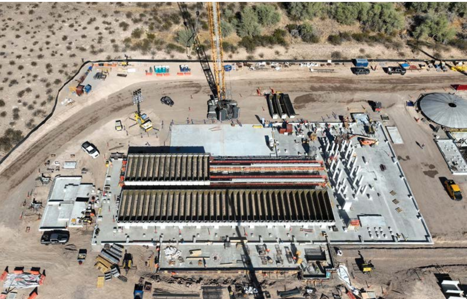
During December 2024, the electrowinning cells were mounted in the electrowinning building in preparation for building erection. (Photo: Taseko Mines)
